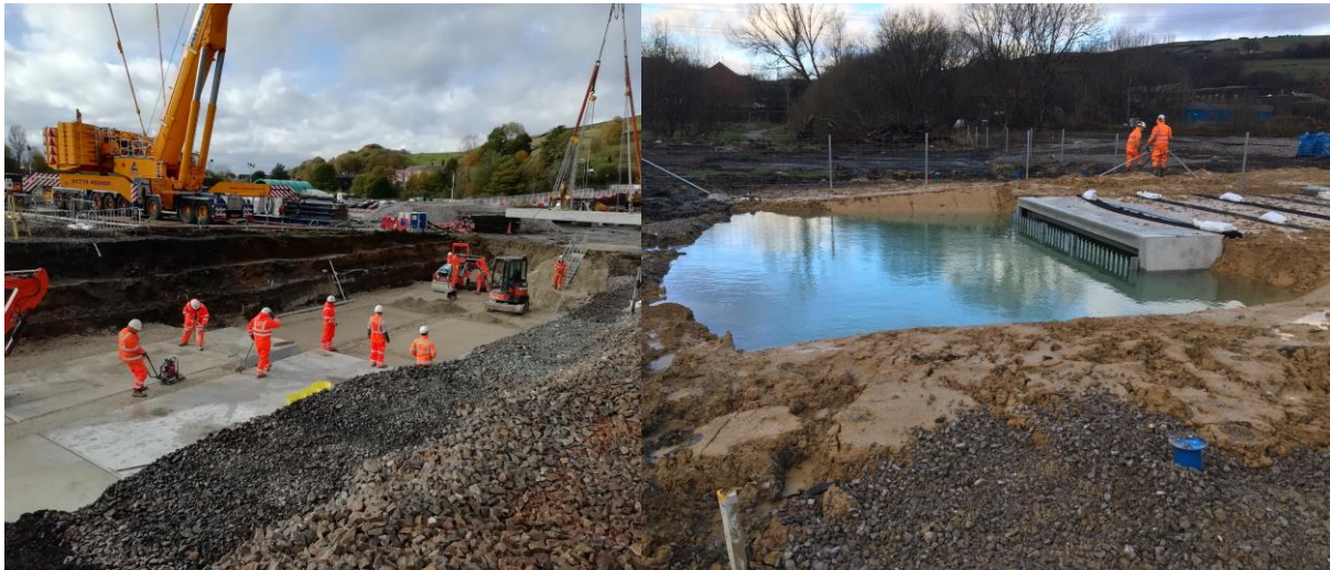
Figure 10: Photos of the box culvert during construction (left), and after construction when the dewatering system was turned off and the groundwater level had rebounded (right).
