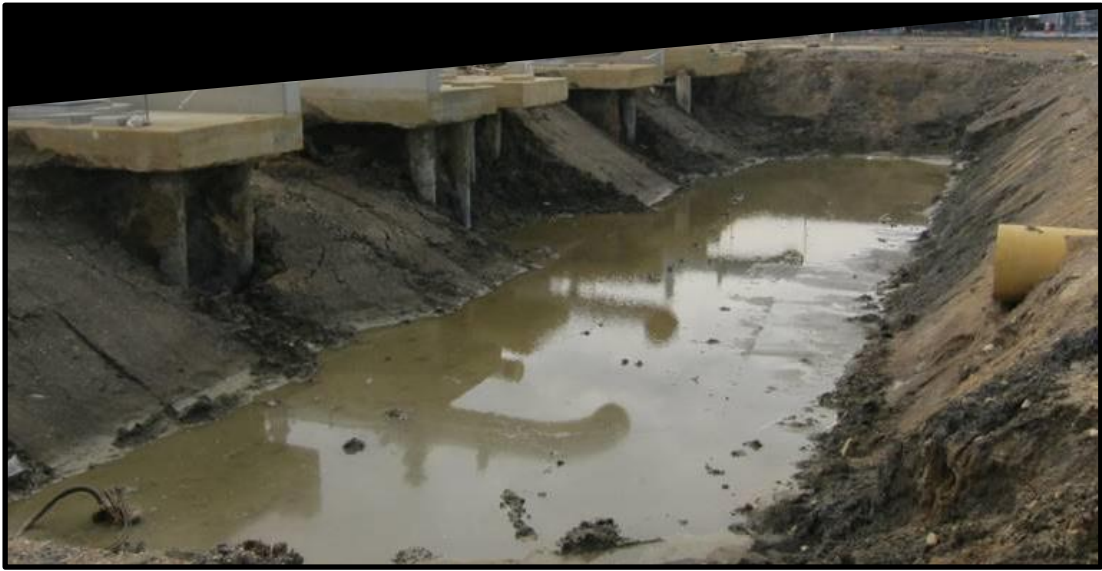
Figure 2. Excavation with soil erosion and unstable sloping sides
