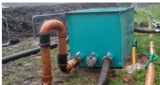
Figure 14. Water holding tank before discharging to the multiple-well recharge system.
