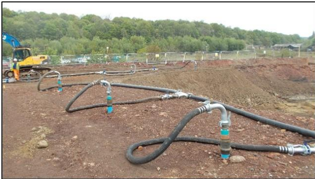
Figure 4. Pressurised wells to recharge abstracted groundwater back to the aquifer.
