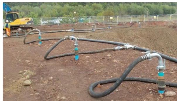
Figure 10. Series of pressurised recharge boreholes.
