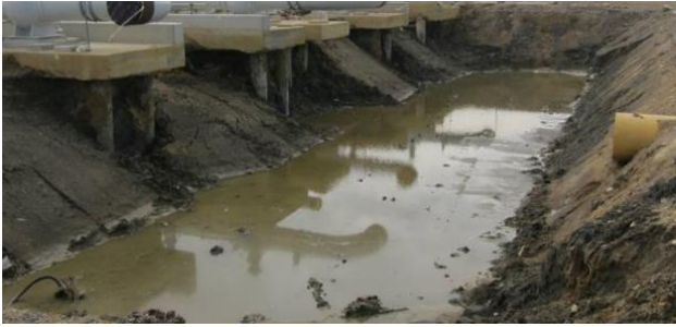
Figure 2. Excavation with unstable sloping sides.
